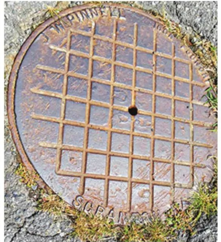
This waste water cover located on Scranton's South Side was produced by the Pinnell Foundry.
